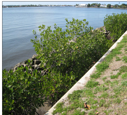
Example of a “redeemed seawall” where mangroves were planted in front of an existing hard structure.
